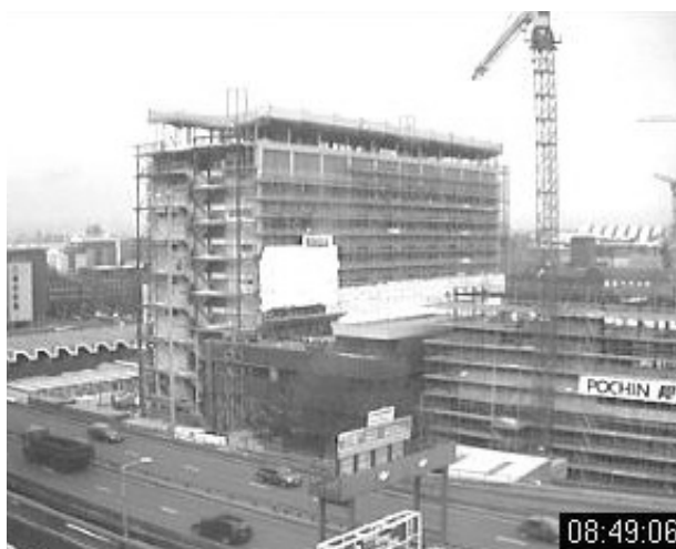
Figure 1: A webcam picture of the main John Dalton laboratory building during its refurbishment. The new central IT building is shown on the right.
